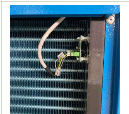
Temperature/humidity electronic board
